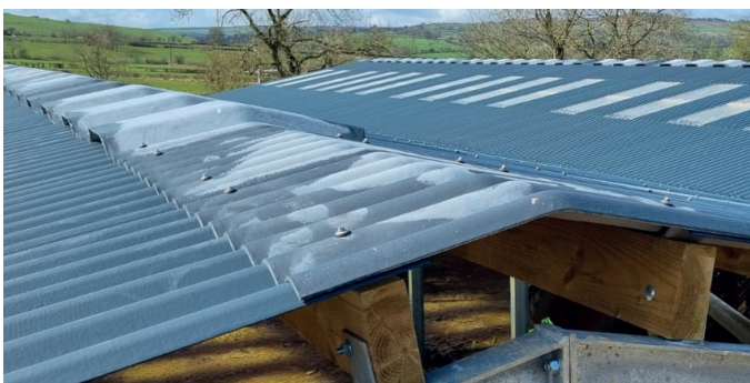
Fig.1 showing Efflorescence on ridges naturally occurring
